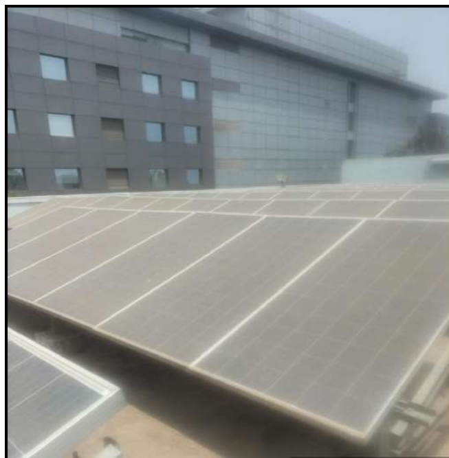
Photograph of Roof Top Solar PV Plant:
