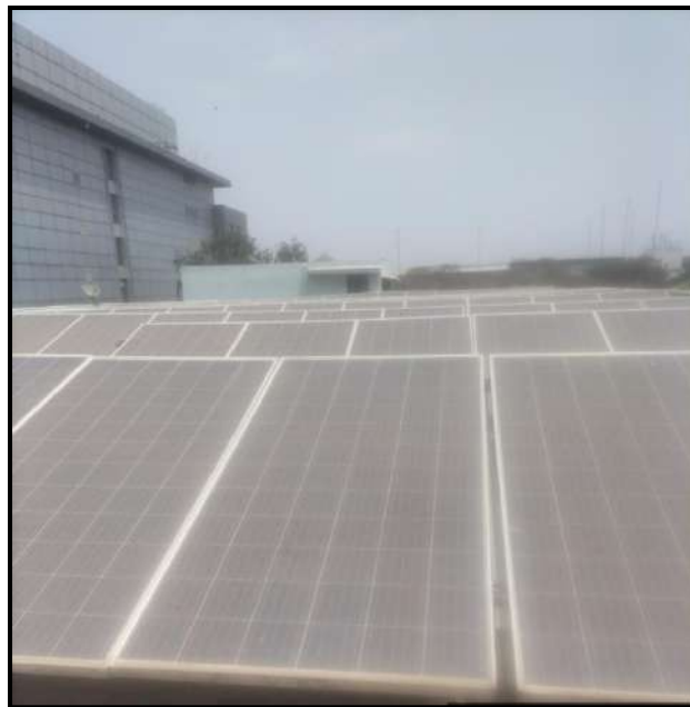
Photograph of Roof Top Solar PV Plant:
